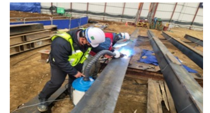
Utilizing dust collection equipment
